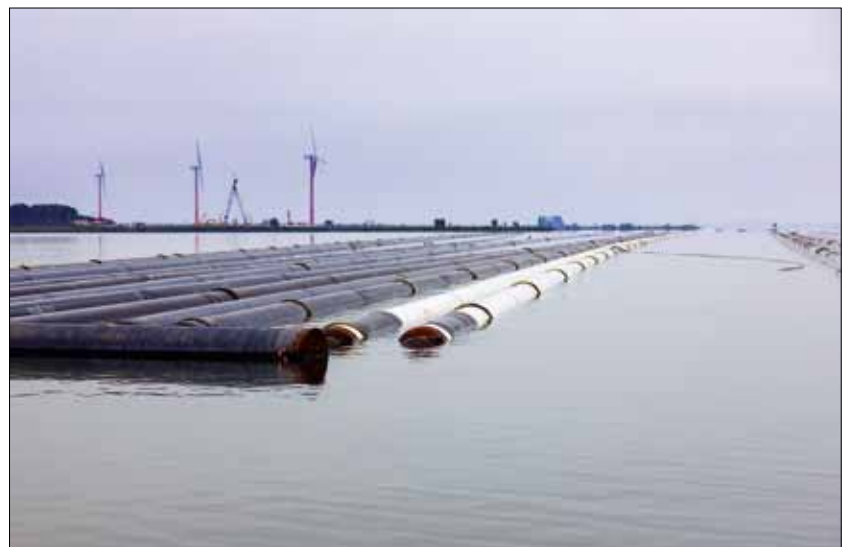
Figure 3. »Parking lot« of the pipelines, which are welded together to partial lengths of 500 to 700 m and sealed at the ends
